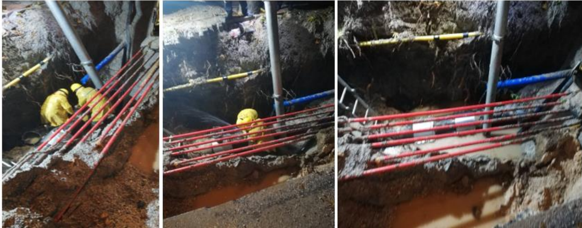
Picture 3. Steel pipe failure
