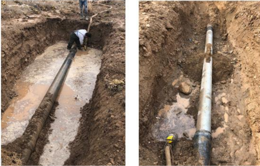
Picture 1. PVC pipe failure
