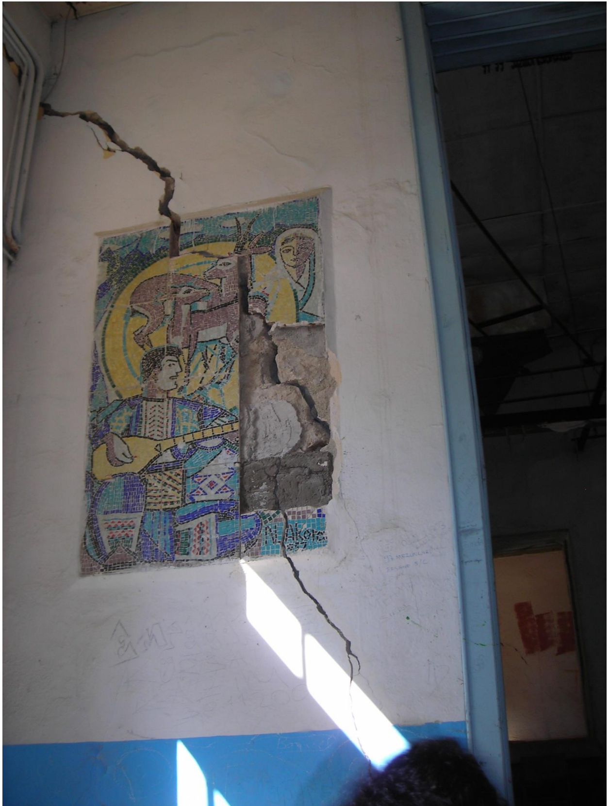
A crack in a theater saloon. The mosaic was made by the students.
